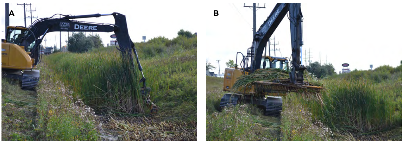
Figure 3. Ditch management with the Herder bucket mower attachment for cutting and removing ditch vegetation.
